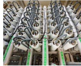
Water Reuse Separation, Feed
